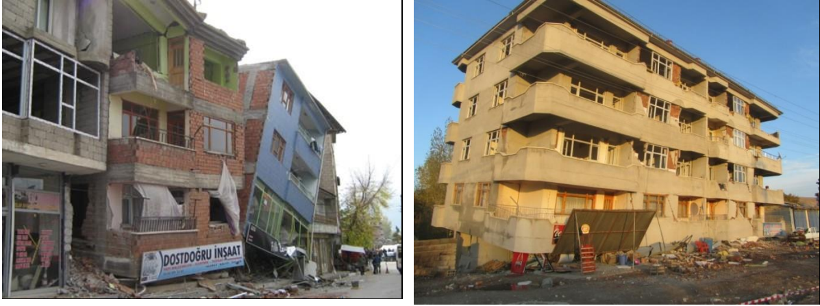
Figure 5. Soft storey damage observed in Van Erciş earthquake
