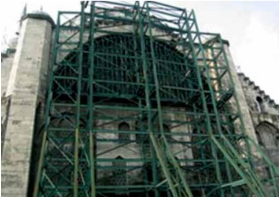
Figure 4. Steel Suspension System in The Main Arch of The Mihrab Façade (Sesigür and Çılı, 2014: 75)
